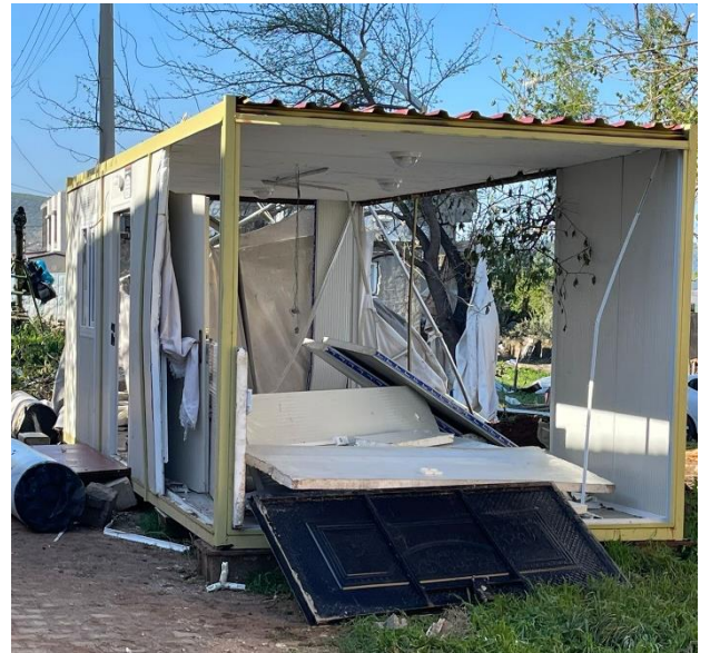
Container destroyed by the storm in Pazarcık district, Kahramanmaraş, province on 20 April 2023. Credit: OCHA.
